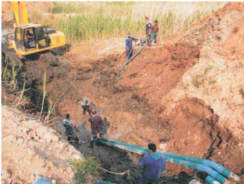
Figure 1: A view of the pipe installation works undertaken in the Kogmanskloof River. The works undertaken in September 2015.
